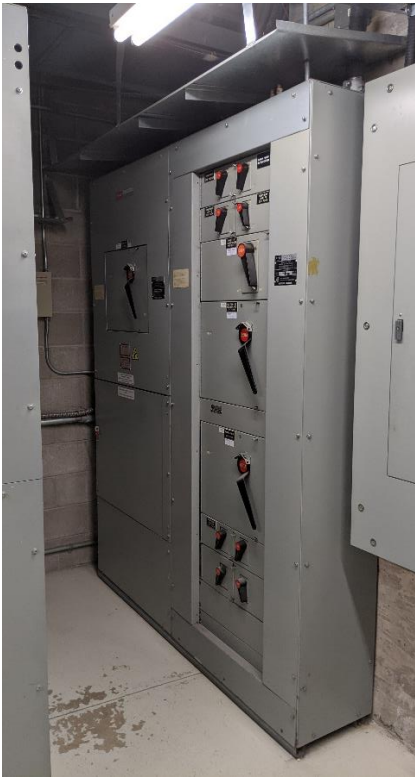
Photo 2: 600Volt main distribution switchboard.
