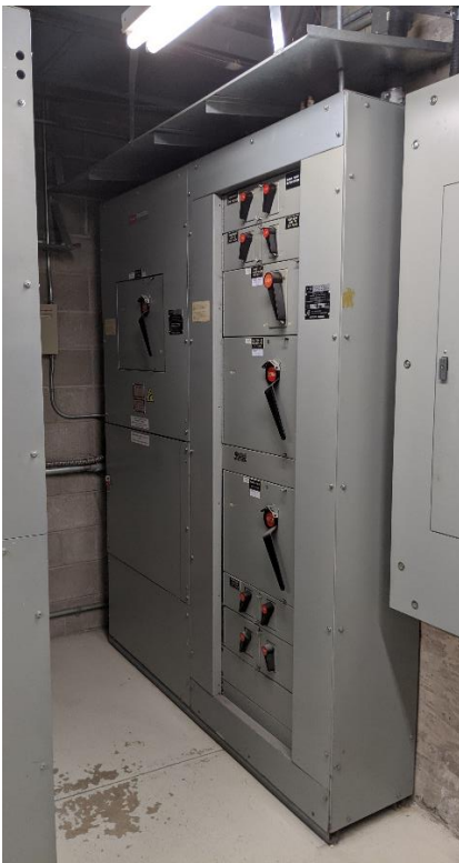
Photo 2: 600Volt main distribution switchboard.
